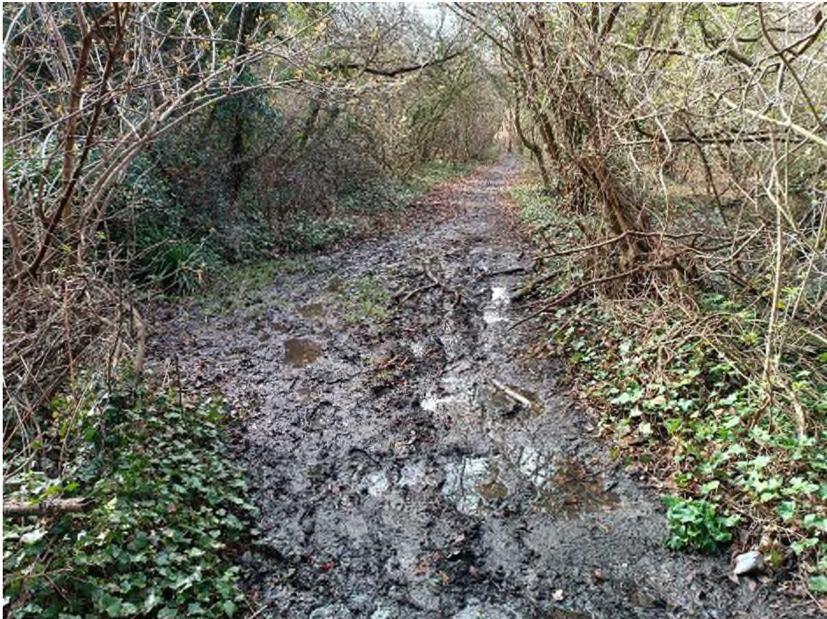
Figure 18 Poor quality path surface between Batchworth Heath and Bishop's Wood
